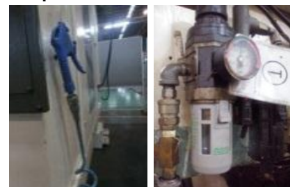
Inspection for Air Gun and Filter
